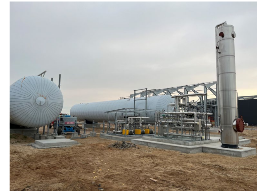
CO 2 -storage tanks
