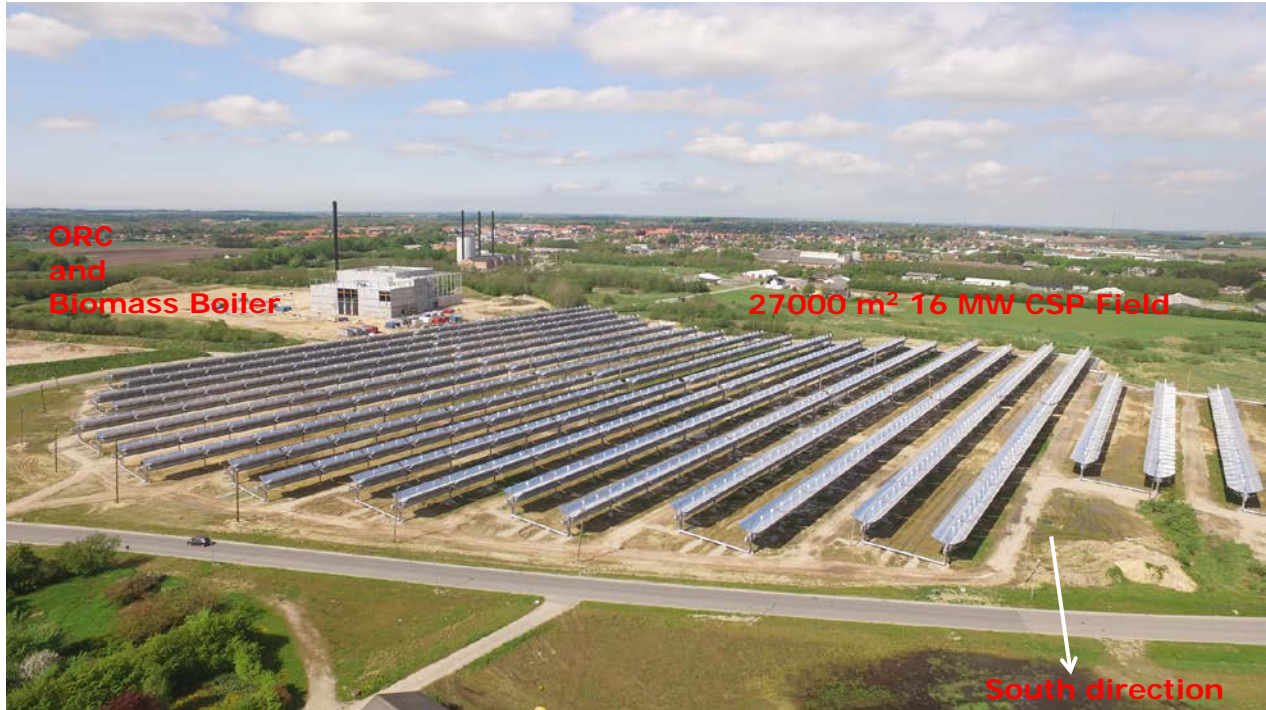
Figure 1. The Brønderslev ORC-CSP biomass combined heat and power plant. The collector area is 27000 m 2 and nominal thermal power 16 MW.
